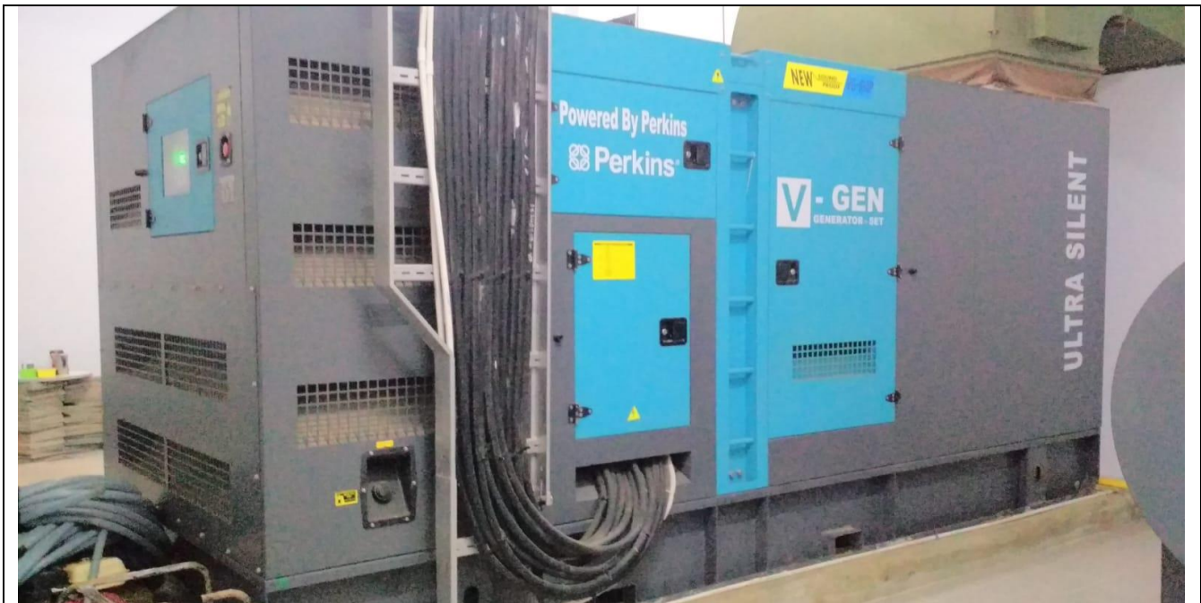
Biodiesel Combined Cooling Heating and Power Integration Unit (Universitas Esa Unggul – Jakarta, Bekasi, Tangerang )
