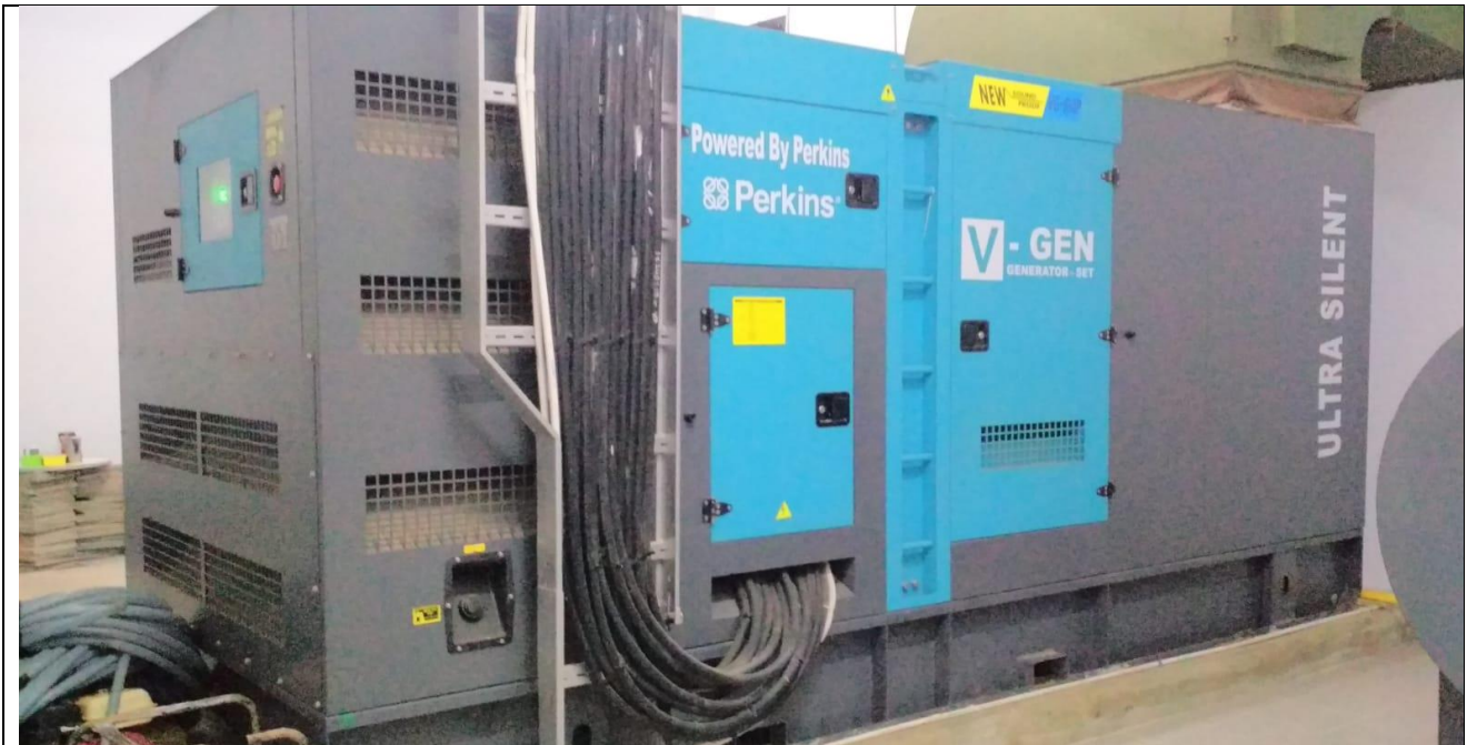
Biodiesel Combined Cooling Heating and Power Integration Unit (Universitas Esa Unggul – Jakarta, Bekasi, Tangerang )
