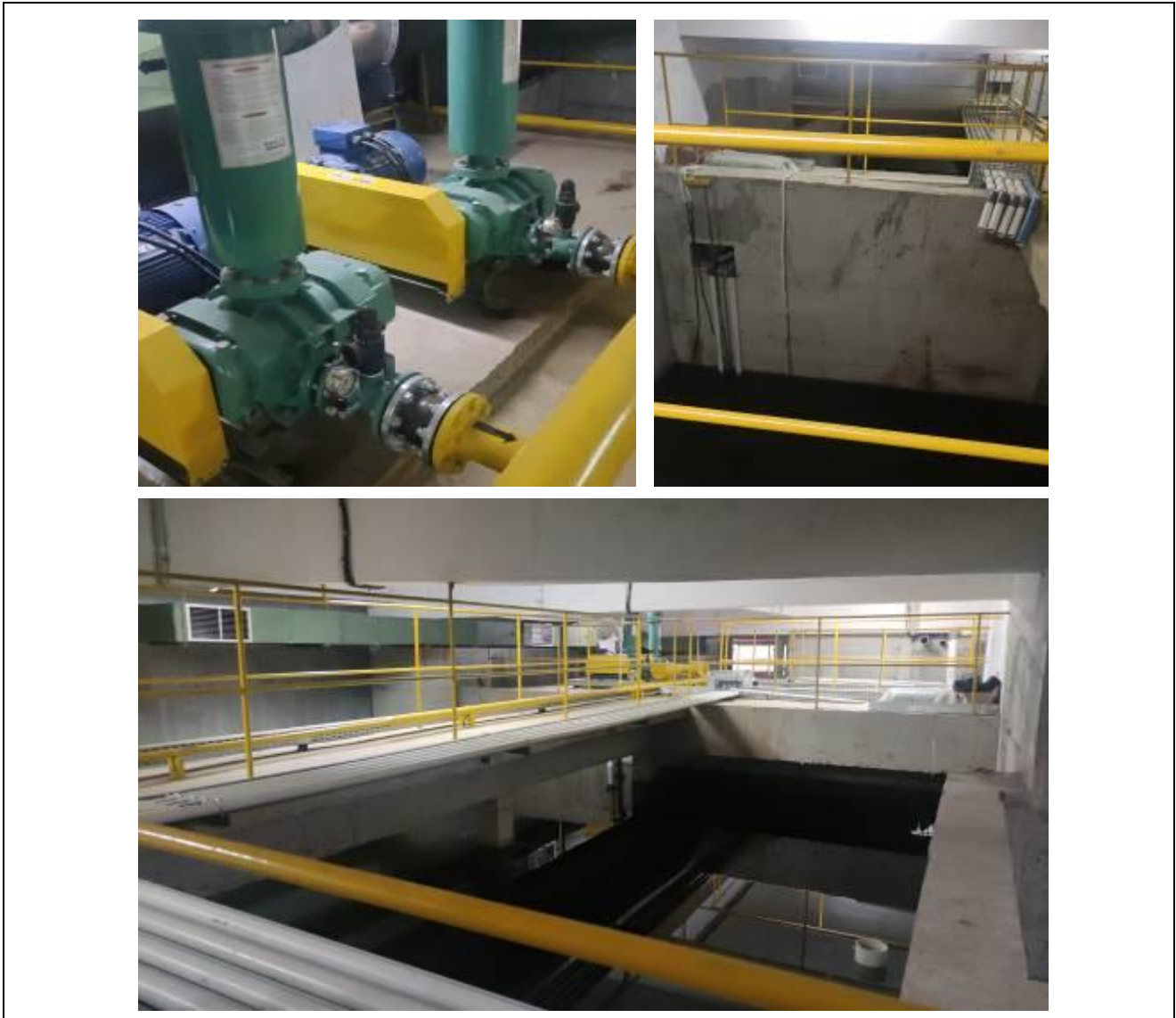
Picture 1. Sewage disposal treatment system in Esa Unggul University
