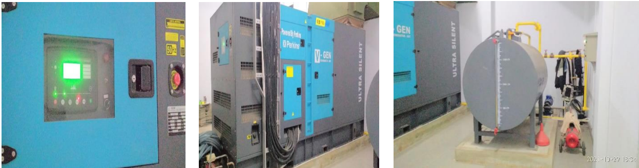
Biodiesel Generator and Power Integration Unit (Esa Unggul University - Bekasi) Esa Unggul University – Bekasi already has a renewable energy source, namely BIO DIESEL with a capacity of 520Kwh that reaches the entire building area as well as the main street lights.
