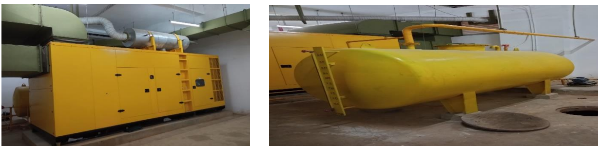
Biodiesel Generator and Power Integration Unit (Esa Unggul University – Cikupa - Tangerang) Esa Unggul University – Cikupa- Tangerang already has a renewable energy source, namely BIO DIESEL with a capacity of 640Kwh that reaches the entire building area as well as the main street lights.
